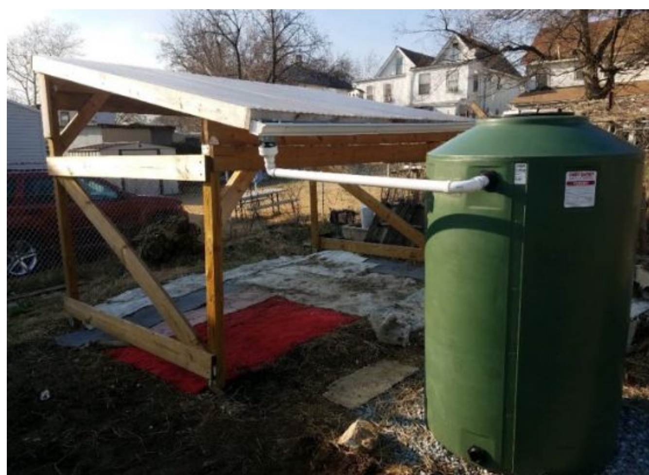
Figure 2: Rain catchment system, Fall 2018
