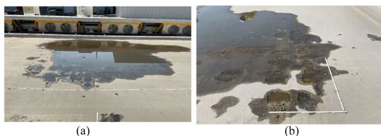
Fig. 8 Visual inspection images from the inspection reports of the testbed (a) Small to large spalls looking east 3,25 m 2 (35 sq.ft.); (b) large spalls looking south 2,32 m 2 (25 sq.ft.)
